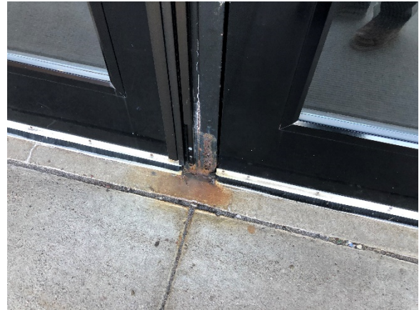
Exterior hollow metal door frame rusting at the bottom.
