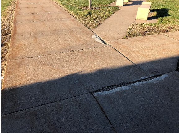
Front entrance sidewalk is damaged and uneven in a few spots.
