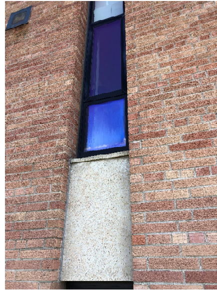
Exterior glazing panel is foggy and should be replaced. A few other window gaskets have come loose and need to be addressed.
