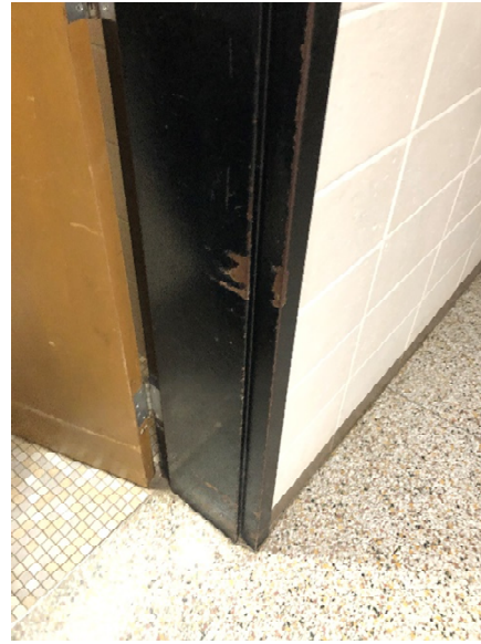
The interior door frames throughout the building are hollow metal frames and are in fair to good condition.
