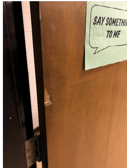
The interior wood doors are showing signs of their age and use. This door like many others have chips and scratches in them.
