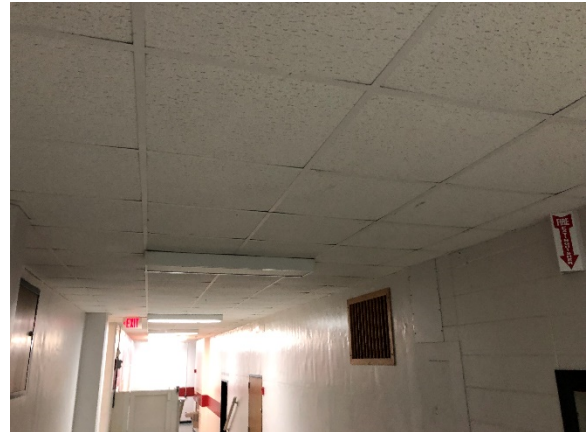
Ceilings on the lower level are mainly 2x2 acoustical ceiling tile and grid. The tiles are sagging from humidity and are chipped and worn.
