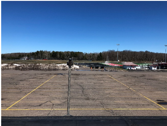
North parking lot. Several areas have been patched in the past. Asphalt is in poor condition.
