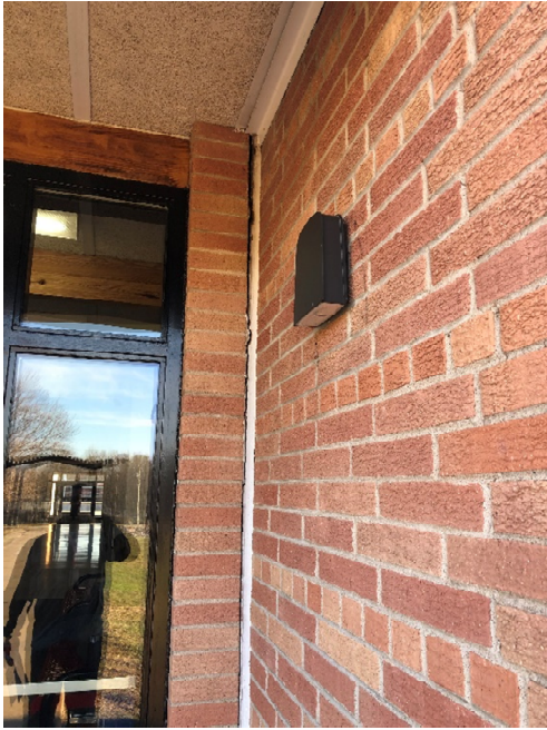
Exterior caulk joint is tearing away from exterior brick and needs to be replaced.
