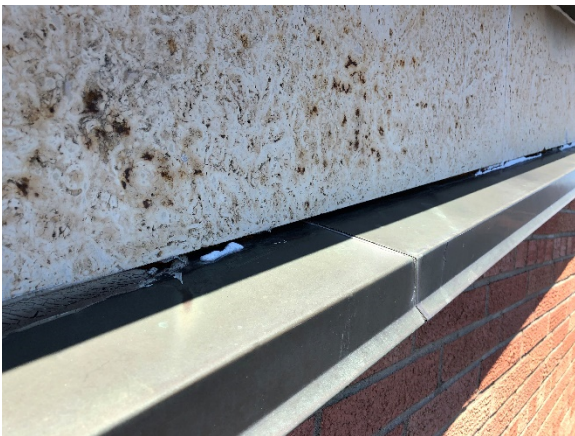
Exterior caulking is missing at the stone band around the gym exterior wall.
