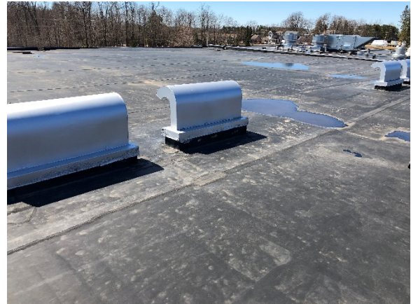
The roofs are in good shape; however, some roofs are nearing their life span (20 years).
