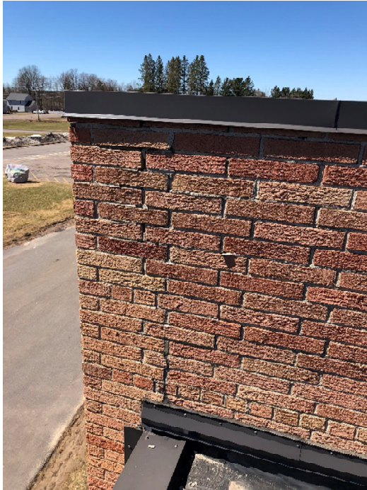
Corner of pool building is cracking and the inside shows signs of water intrusion.
