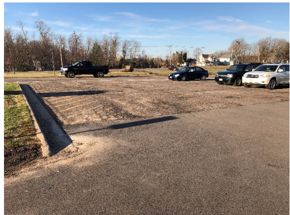
West parking lot asphalt is in poor condition and crumbling.
