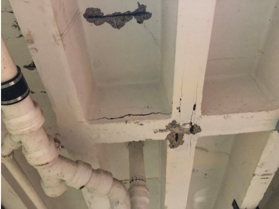
Concrete reinforcing part of the main level floor structure is exposed and in need of repair.
