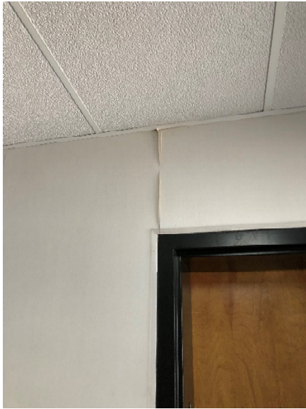
This picture shows the seam coming apart on the vinyl wall covering in the 1996 addition.
