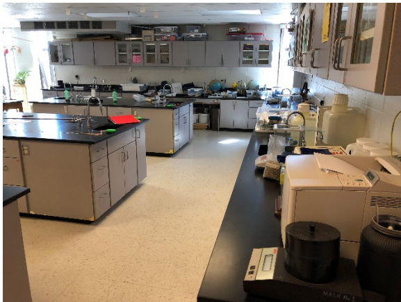
The casework installed in the 1996 addition and art classrooms are chipped and damaged in areas.
